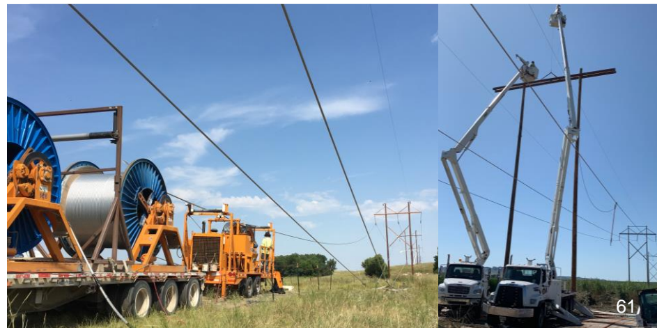
175-mile electric transmission line - Rapid City to Stegall, Nebraska
