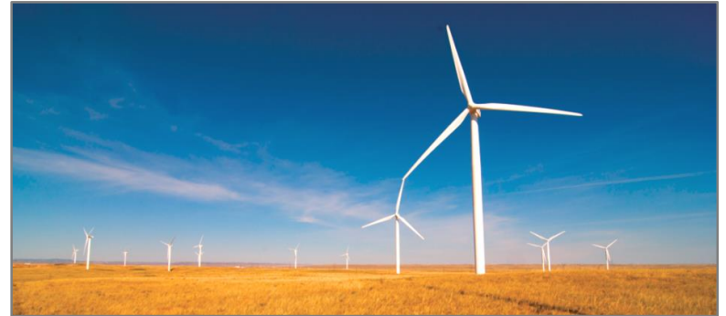
Pictured: Happy Jack Wind Farm located near Cheyenne, Wyoming, serves Wyoming and South Dakota Electric (owned by Duke Energy)
