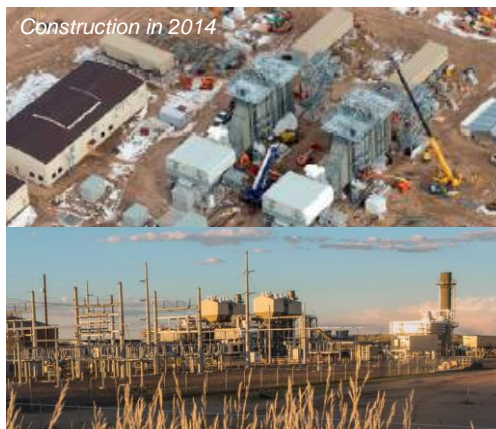
Cheyenne Prairie Generating Station
