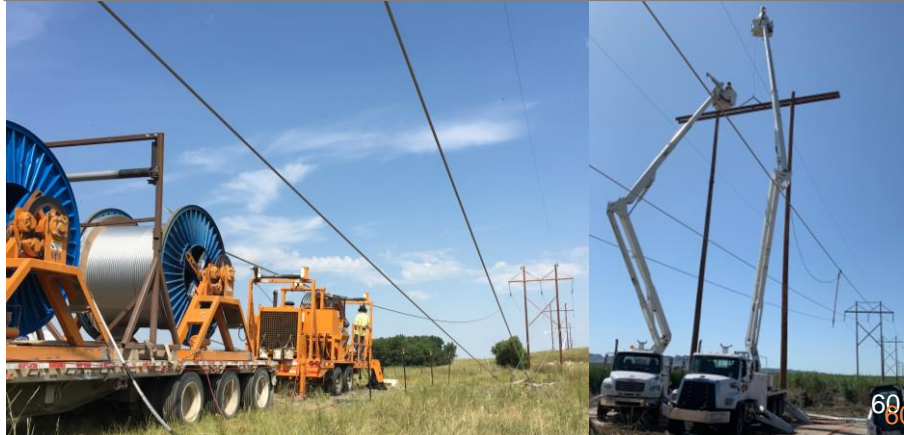
175-mile electric transmission line - Rapid City to Stegall, NE
